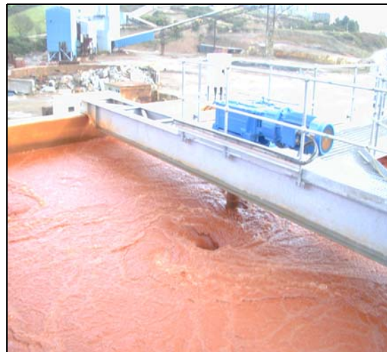
Figure 5. Stage II reactor mixer bridge
